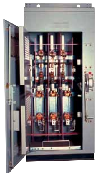
Interior View of Switch/Fuse Bay
