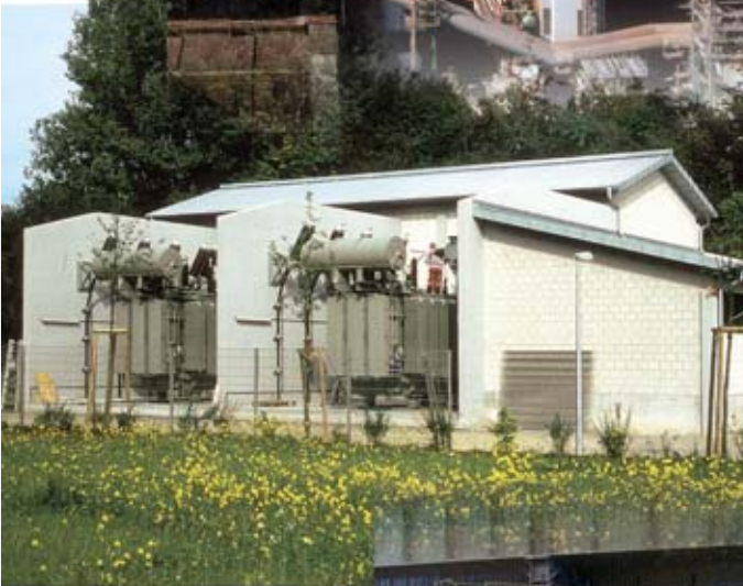
Application Public power supply system
