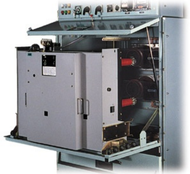
The circuit breaker in withdrawn position
